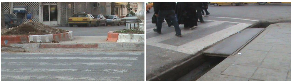
Figures 11 and 12: Street has a level that wheelchair users couldn't go across the street.
