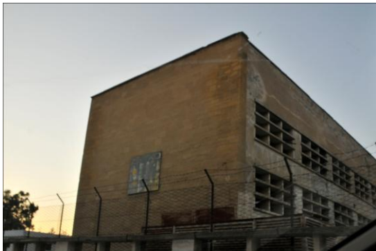
Figure 7: Abandoned Industrial Building
