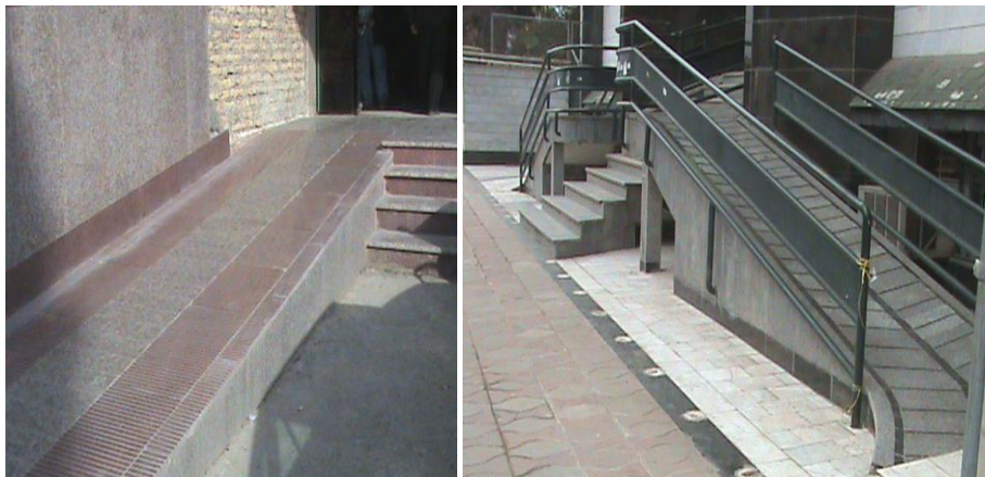
Picture 4: An entrance to a general hospital, the slope of ramp is not standard and is unprotected border. Picture 5: Ramp of inappropriate slope for access into a clinic.
