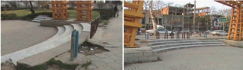
Figures 5 and 6: Park has stairs and bollards. There isn't any ramp for the disabled.
