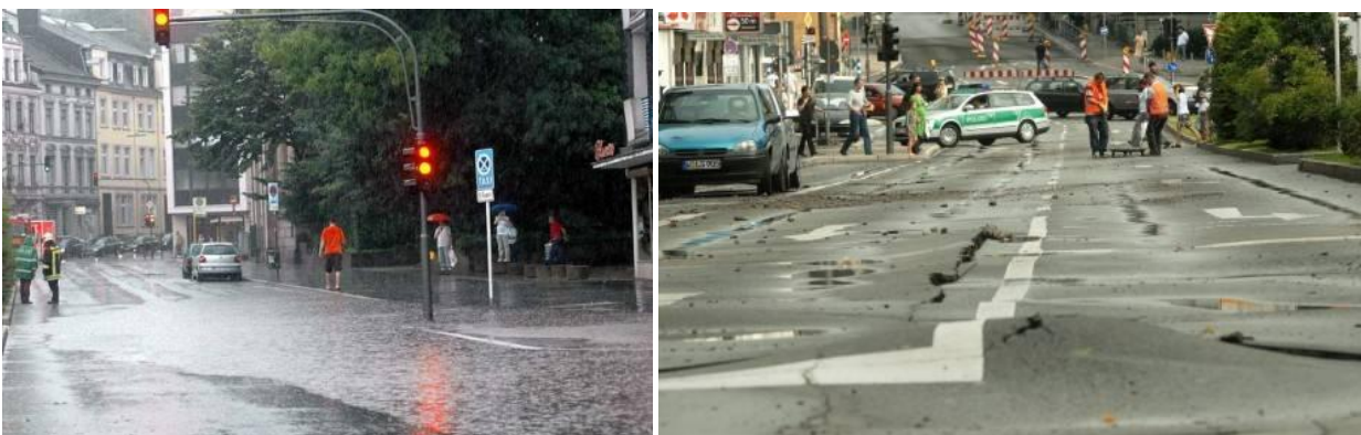
Figure 4: Damage due to uncontrolled storm water run-off.
