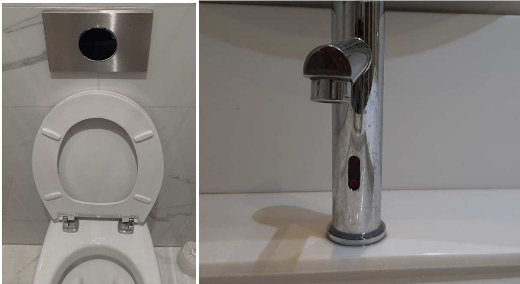
Fig. 2: Ultra-Low Flow plumbing fixtures (Source: Author, 2021)
